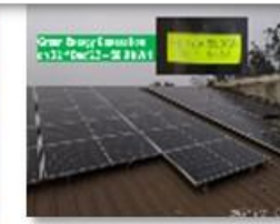
Solar Plant 15 kWp at M/s ZF India
