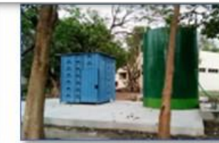
Bio-Gas Plant, 250 kg/day at M/s Timken
